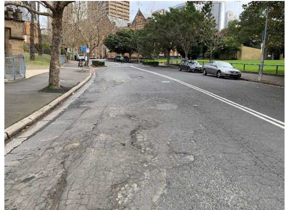
Condition 5 – Very Poor
