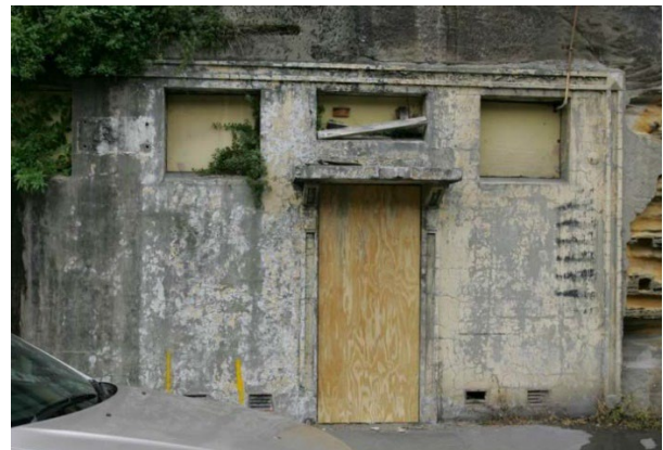
Condition 5 (very poor)
